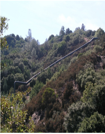
Steam line descending from the West Coleman Pad
